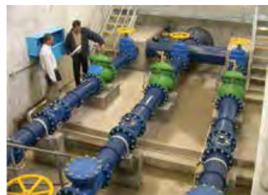
Above: External view of the Khayelitsha pressure management installation, (© City of Cape Town); Khayelitsha pressure management installation, (© WRP (Pty) Ltd)
